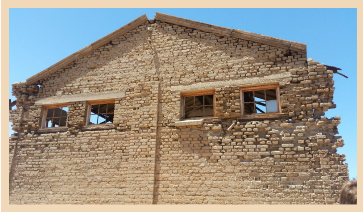
Figure 86 Advanced weathering of a historical mining building
